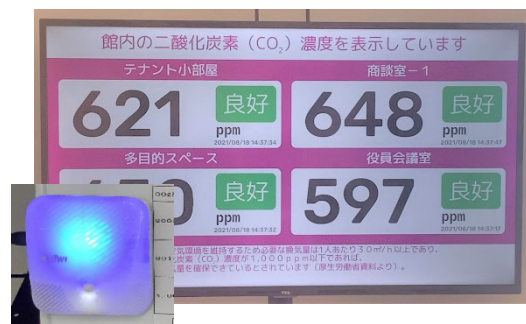
Light with alarm CO 2 concentration in the room can be confirmed on the monitor
